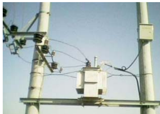
Figure 1. Distribution transformer in rural power network of China
