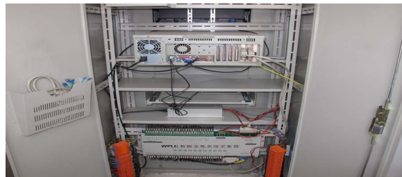
Fig. 3 Inner station concentrator of data acquisition system
